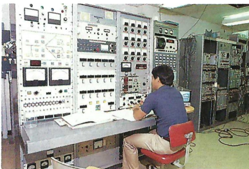
Accelerator control panel in the Nuclear Science Center
